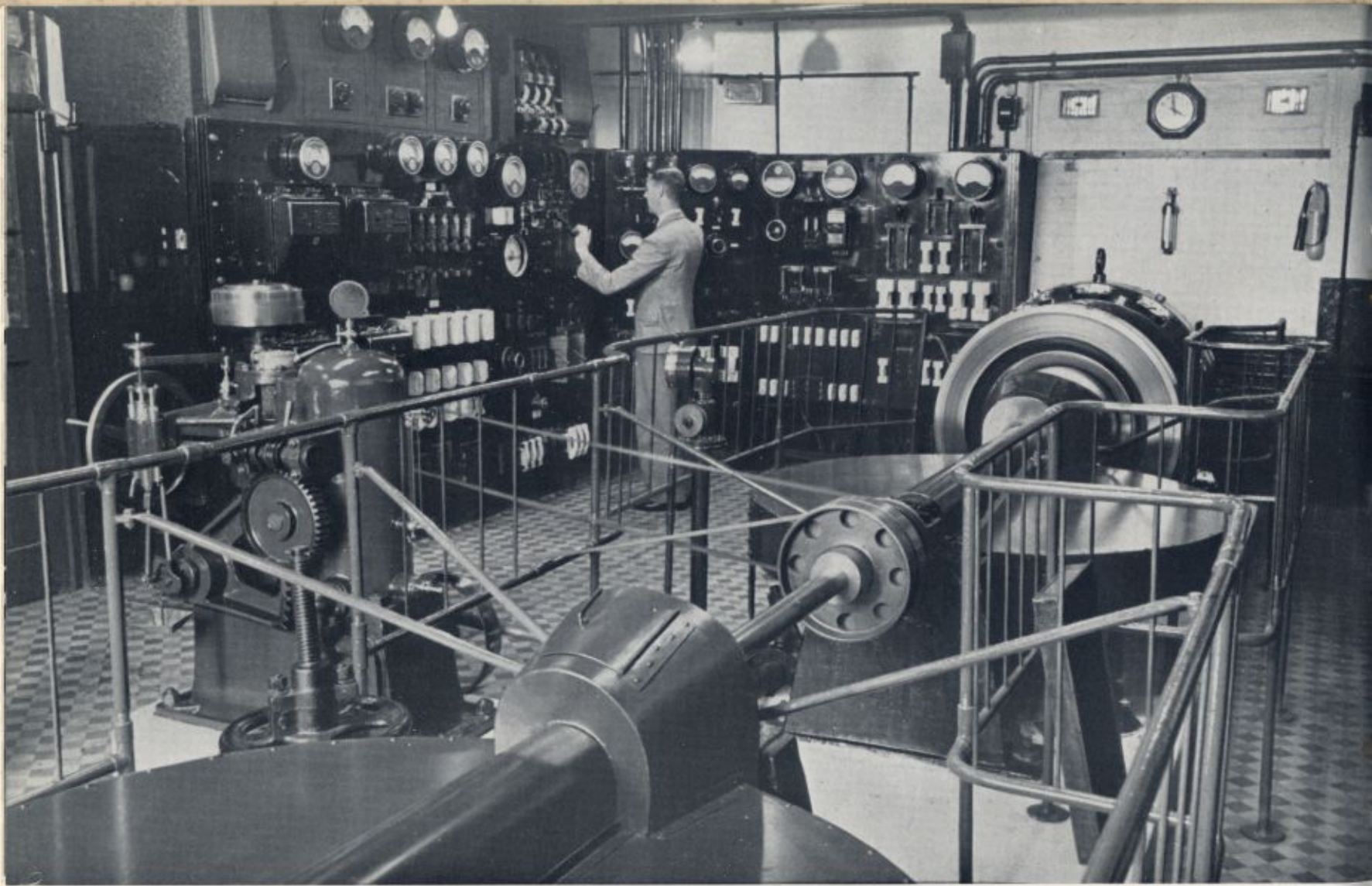
POWER CONTROL SWITCHBOARD
